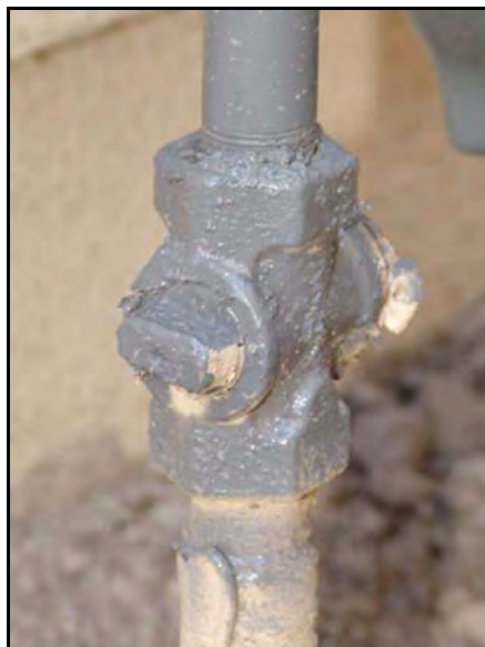
Main Shut-Off "OFF"
