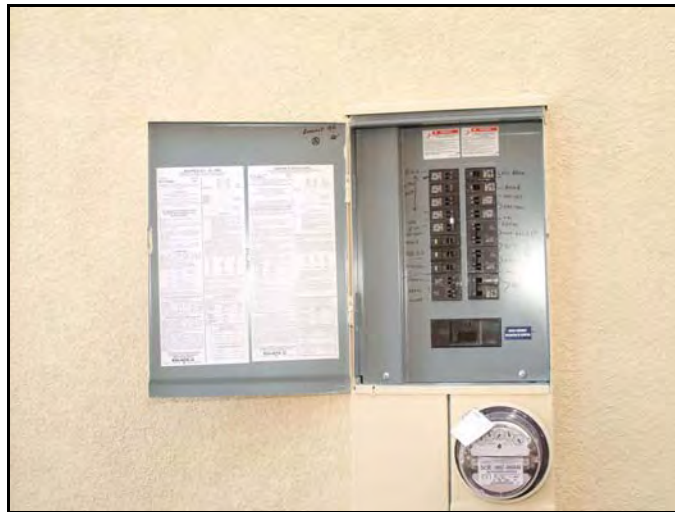
Electric Meter: Typically located outside of home near front.
