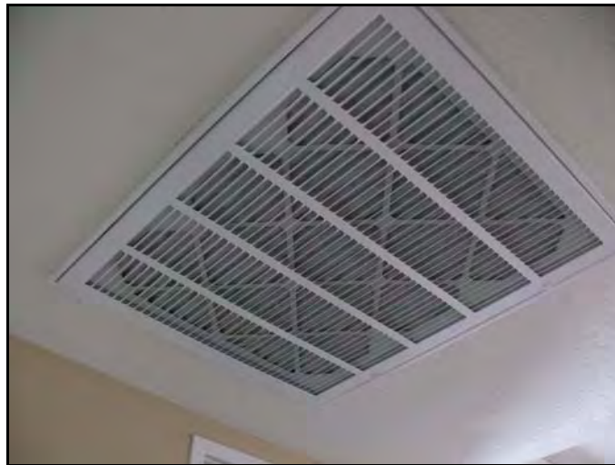
Example of an Air Filter Location
