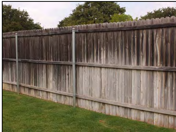
Example of the Effects of Sprinklers on Wood Fencing
