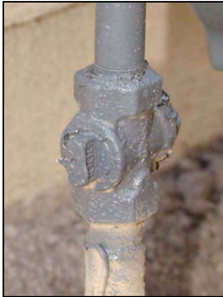
Main Shut-Off "ON"
