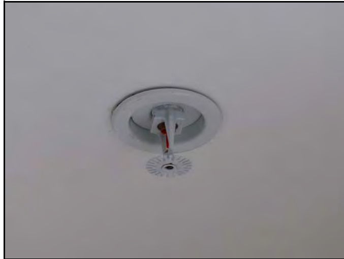
Exposed Fire Sprinkler Head
