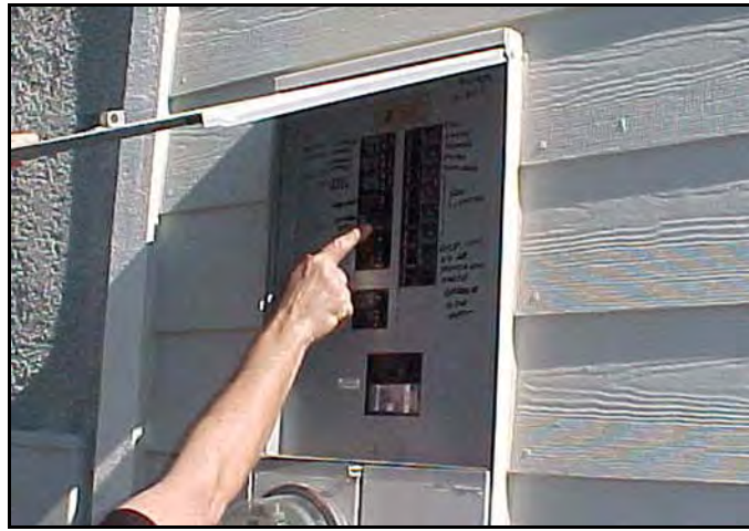
Exterior Circuit Breaker Panel
