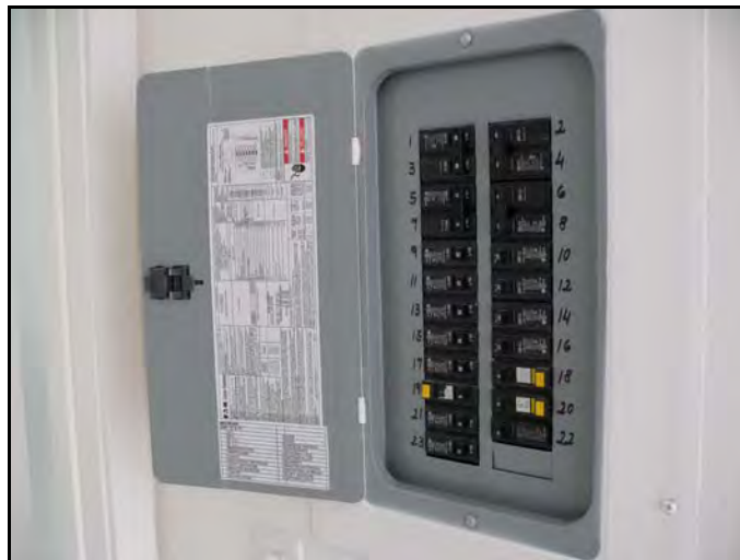
Interior Circuit Breaker Panel
