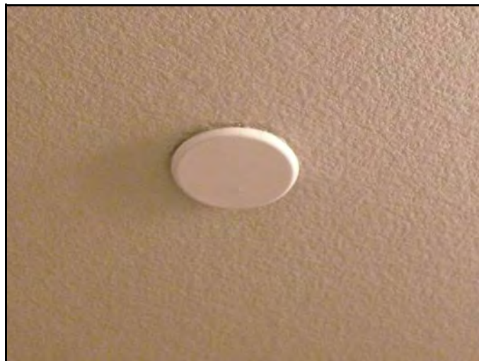
Recessed Fire Sprinkler Head
