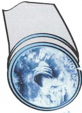
Overflowing cleanout pipe located on private property
